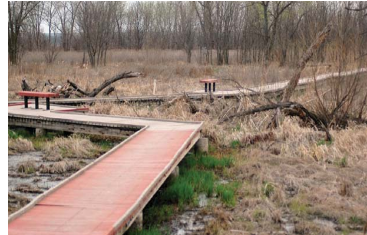
Raised boardwalks protect retention pond areas while allowing users to visit them.
